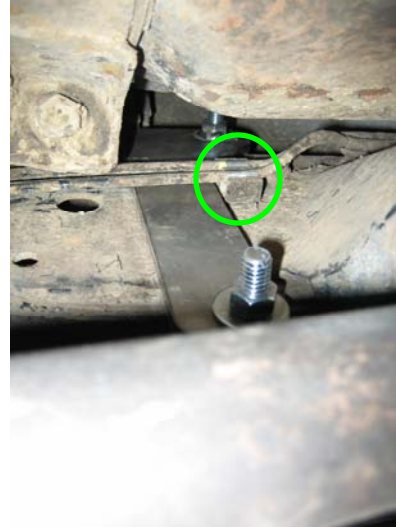
Fig 2 - Inside rear Driver's side frame rail
